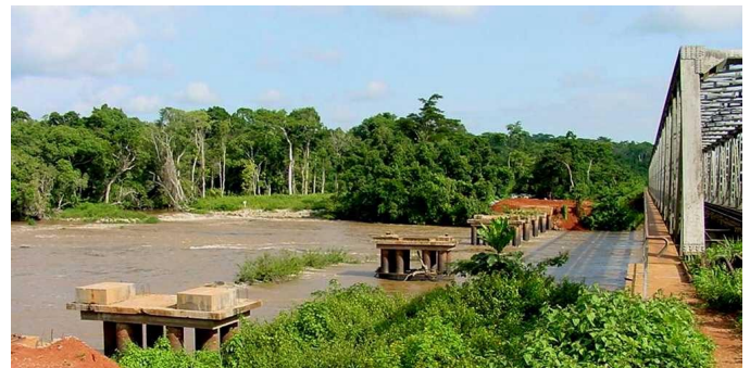
Figure 4D. Removal of a temporary bridge over a river in an induced access management area (pre-existing railway bridge appears on the right).
