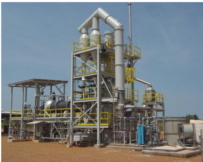
Figure 9C. The hazardous waste-capable incinerator at the Komé Waste Management Facility.
