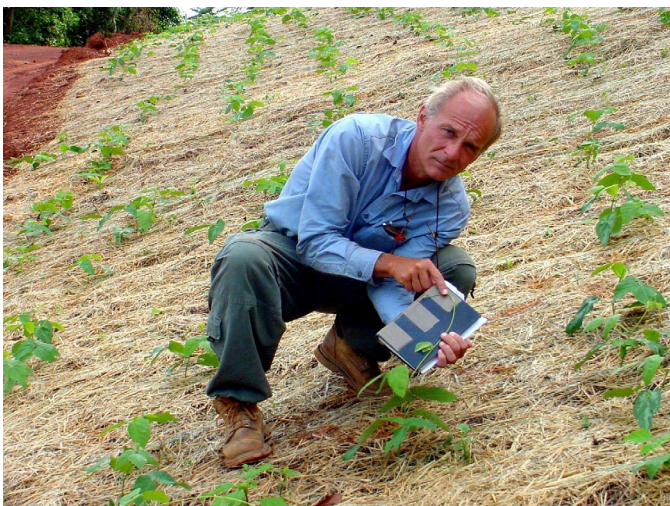
Figure 5C. In certain locations, seedlings were planted in vegetative matting to enhance erosion protection.
