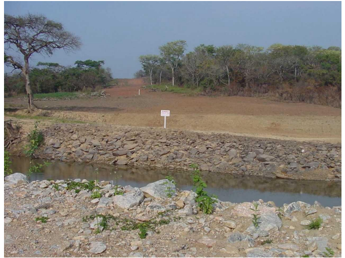
Figure 5D. Rip-rap was used at major river and stream crossings for bank stabilization and erosion control purposes.
