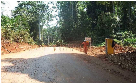
Figure 4B. Guarded checkpoint on a pipeline easement access road in an induced access management area during construction in the area.
