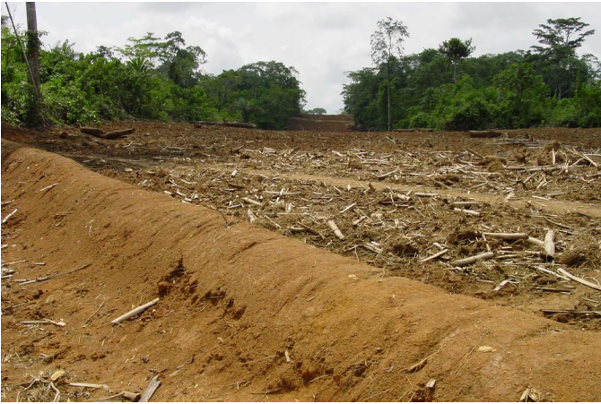
Figure 5A. Earthen berm and chipped vegetation placed on the reclaimed easement for erosion control purposes.
